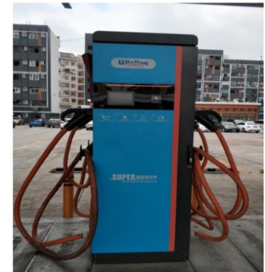
Charging terminal with four chargers
